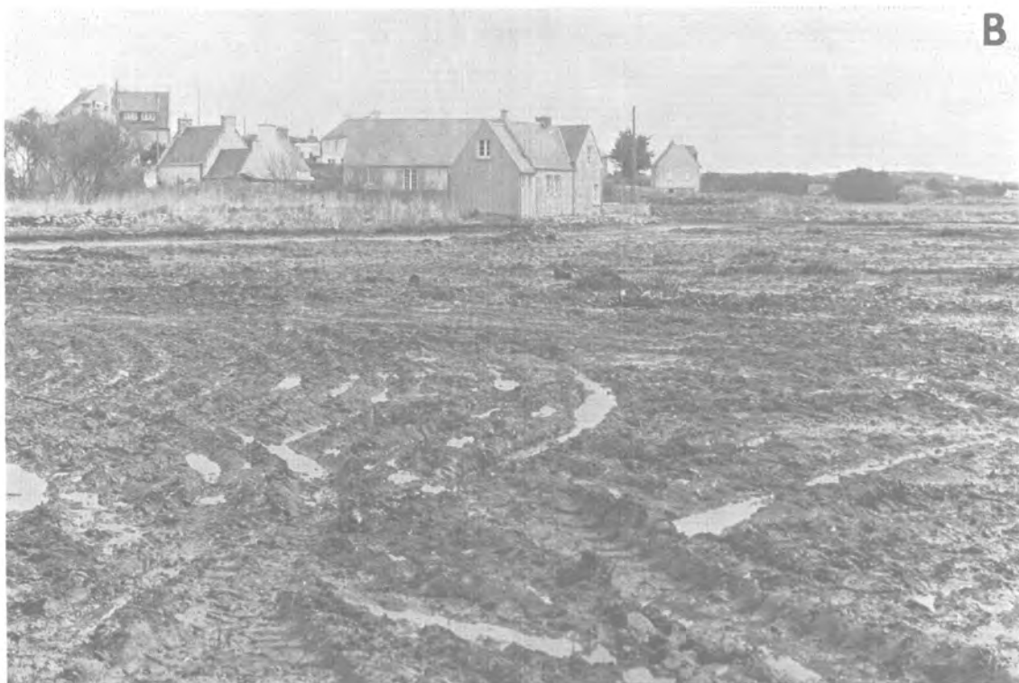
Figure 4-60. (A) High-pressured hosing of the Ile Grande marsh on April 25 (station F-134). (B) The use of heavy machinery on the tidal flat at Ile Grande tended to churn up much of the area and mix oil deep into the sediment (station F-133, April 25).
