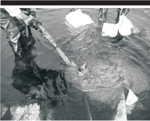
Figure 4. High-pressure flushing and oil recovery from subtidal sands at the Swanson Creek oil spill.
