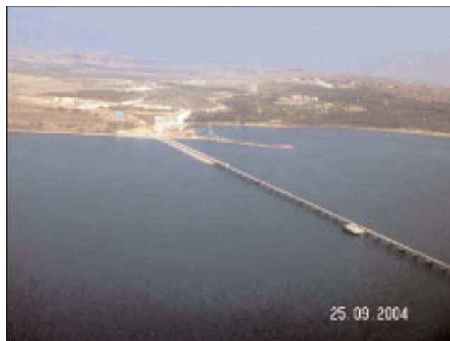
FIGURE 5. OVERVIEW OF CEYHAN MARINE TERMINAL AND THE EXPORT JETTY UNDER CONSTRUCTION (25 SEP 2004). THE JETTY CONTINUES FOR APPROXIMATELY 1 KM (>0.6 MI) TO THE BERTHING AREA (OUT OF THE PHOTOGRAPH). PHOTOGRAPH BY BARBAROS CELIKKOL.
